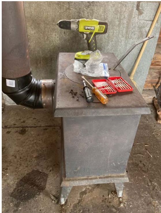
Left: Hubey, Trish, and Darren with chainsaw, clippers, and a hoe to clear water bars Right: Replacing the rusted stovepipe elbow at Spruce Peak Cabin.
