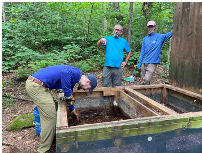
CT Section Trails chair Joe Conaci repairing Story Spring privy bin with Kevin Breton and GMC Staffer Gavin July 2025
